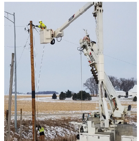
Tony Sienknecht, line foreman; Eric Freese, first class lineman; Aaron Bird, first class lineman; Karl Nielsen, first class lineman; and Tyler Thomas, apprentice lineman, replace a pole that was found to be bad during the pole testing process.
